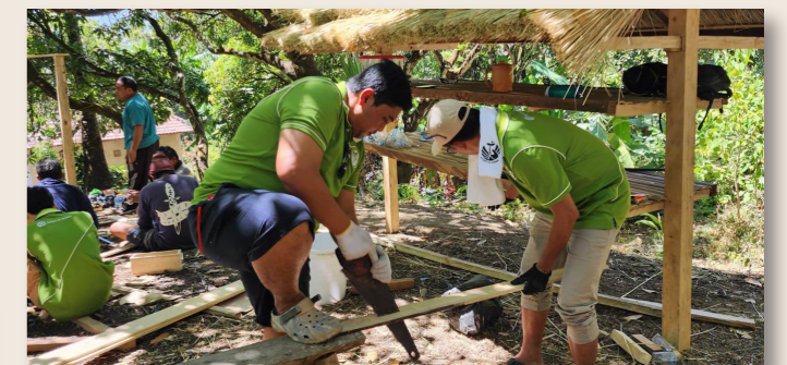
Volunteers sawing wood pallets to build a beehive shelter for placing bee boxes.
